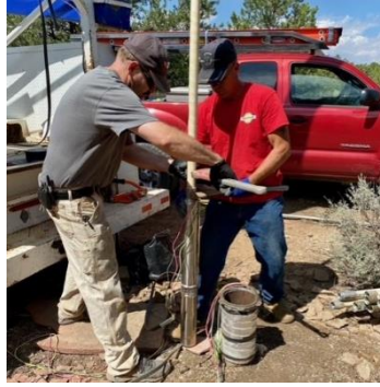
Workers replace a broken well pump for a Self Help client, a single dad from Taos; we got a special grant to pay for the repair. He joined in the work to reduce labor costs and took this photo of his crewmates.
